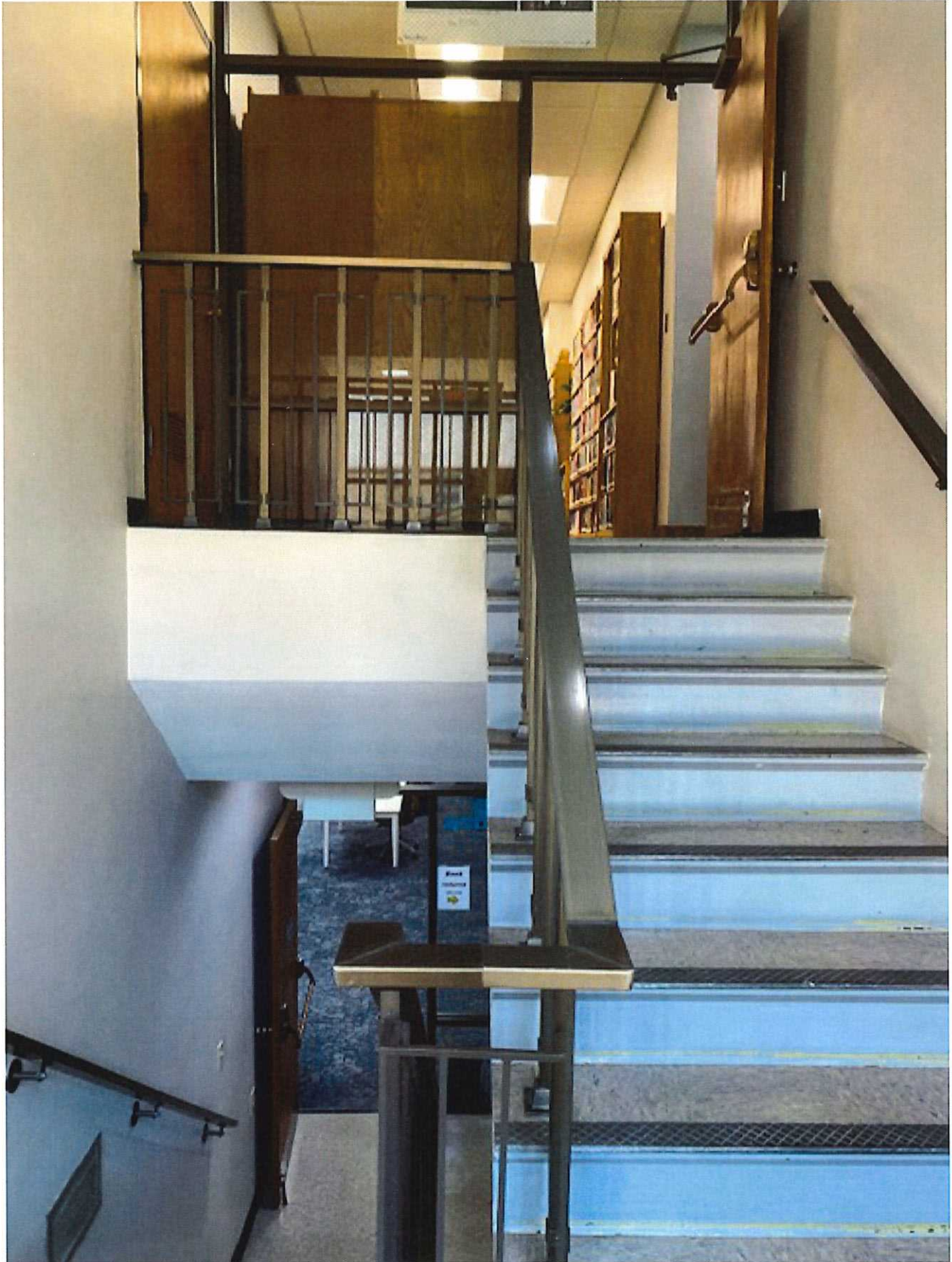
Rear ADA entrance. not to code 6" below height.
